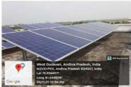
SOLAR PANELS ON FED DEPARTMENT
