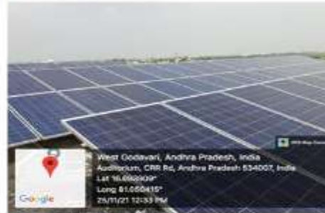
SOLAR PLANT ON IT DEPARTMENT
