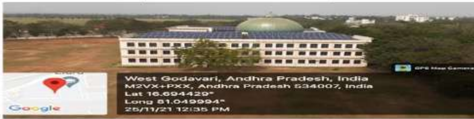
SOLAR PLANT ON CENTRAL LIBRARY
